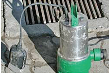
Photo 15: pompe de relevage (AGRIDEA).
